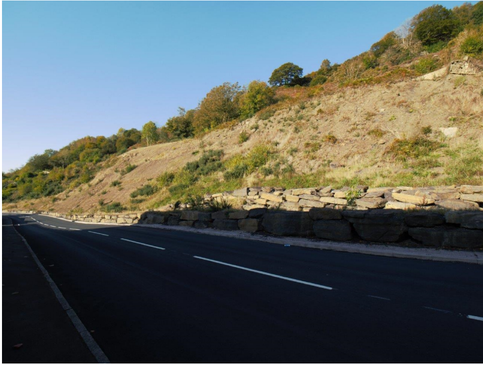
Plate 13: New Gully / Drainage
